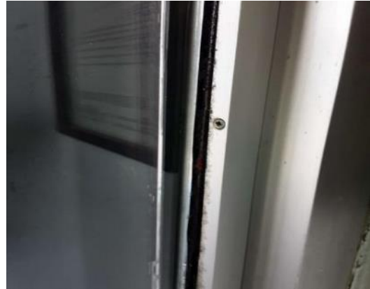
S0009C (None), Other, Caulking, Foyer (Location #: 15)
