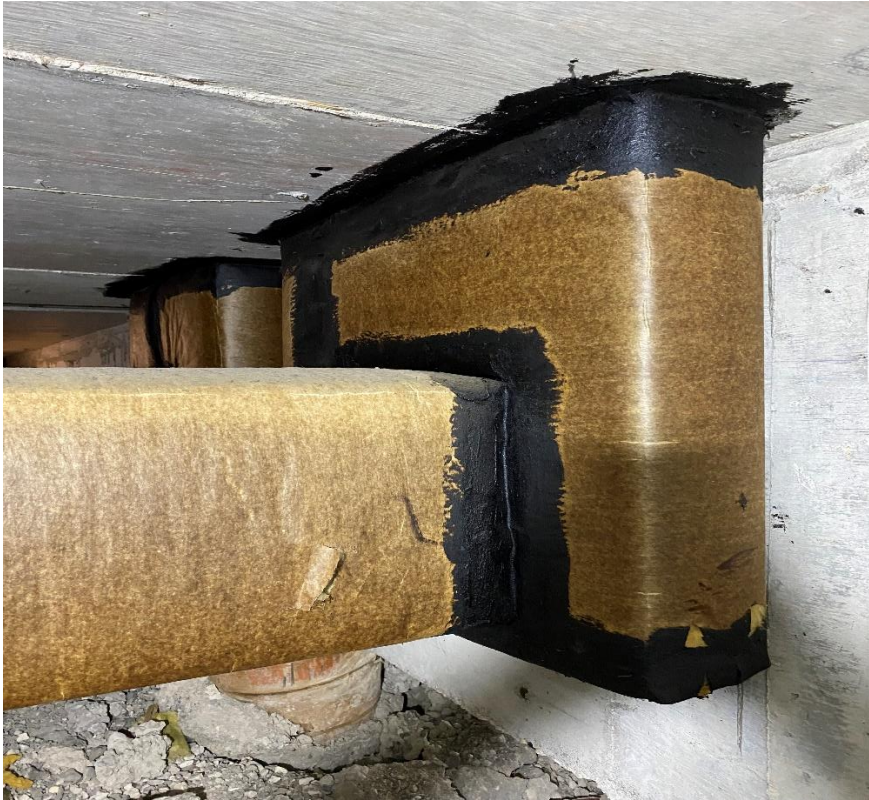
V9000, (Asbestos), Duct, black mastic, Crawlspace (Location # 22)
