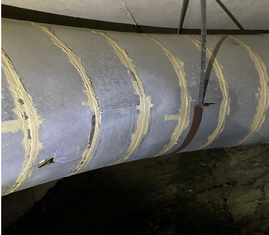
V9000, (Asbestos), Duct, beige mastic, Crawlspace (Location # 22)
