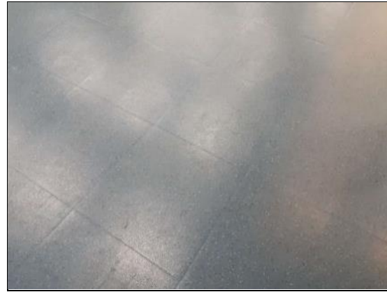
V0000 (None), Floor, Matt Flooring, Foyer (Location #: 15)
