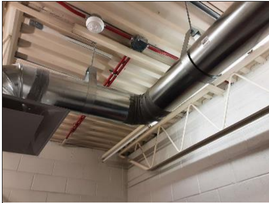
V0000 (None), Duct, Mastic, Grey, Storage Room (Location #: 3)
