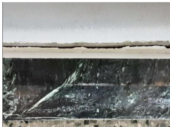
S0007C (None), Wall, Base, Thin-Set Behind, Foyer (Location #: 15)
