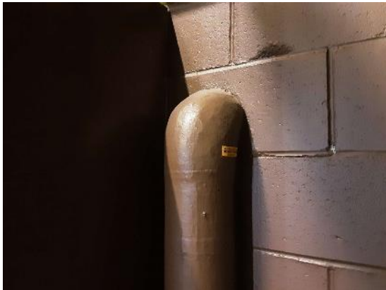
V9000 (Confirmed Asbestos), Piping, Parging Cement, Stage (Location #: 2)
