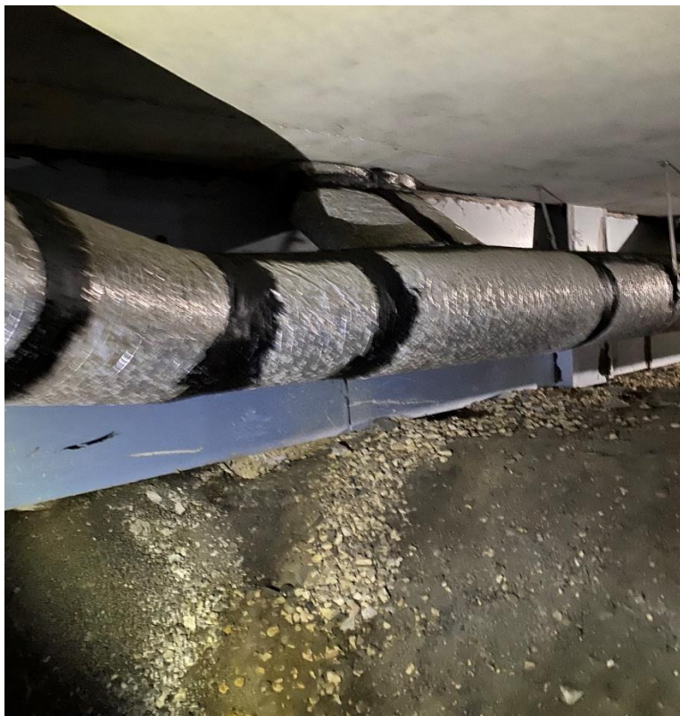
V9000, (Asbestos), Duct, black mastic, Crawlspace (Location # 22)
